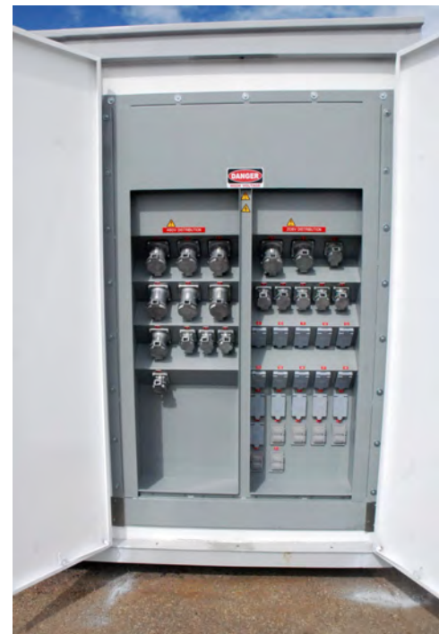
408V/208V External Distribution Panel of a Skid Shack Package
